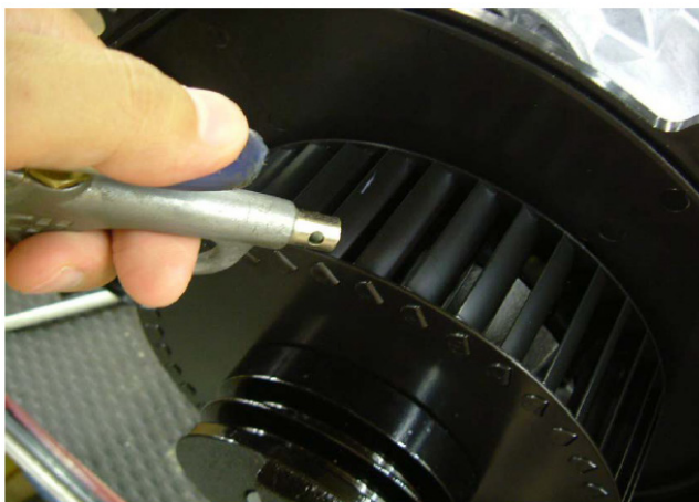
Figure 107: Using compressed air to remove dust from the cooling fan
